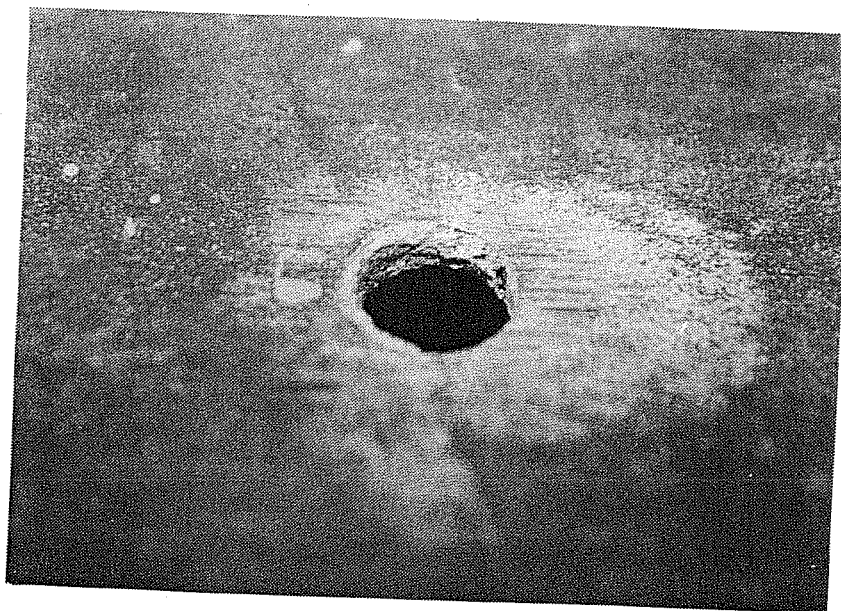
Figure 4.6 Surface abrasion on steel section
